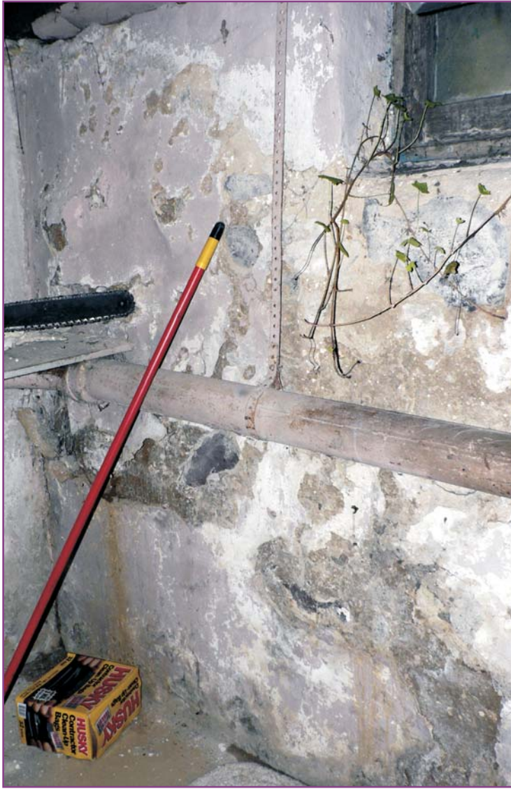
Photograph 38 of 46. Detail of the basement's northern corner showing vegetation entering through the three-light sash basement window and efflorescing moisture damage to the plastered stone foundation walls.
