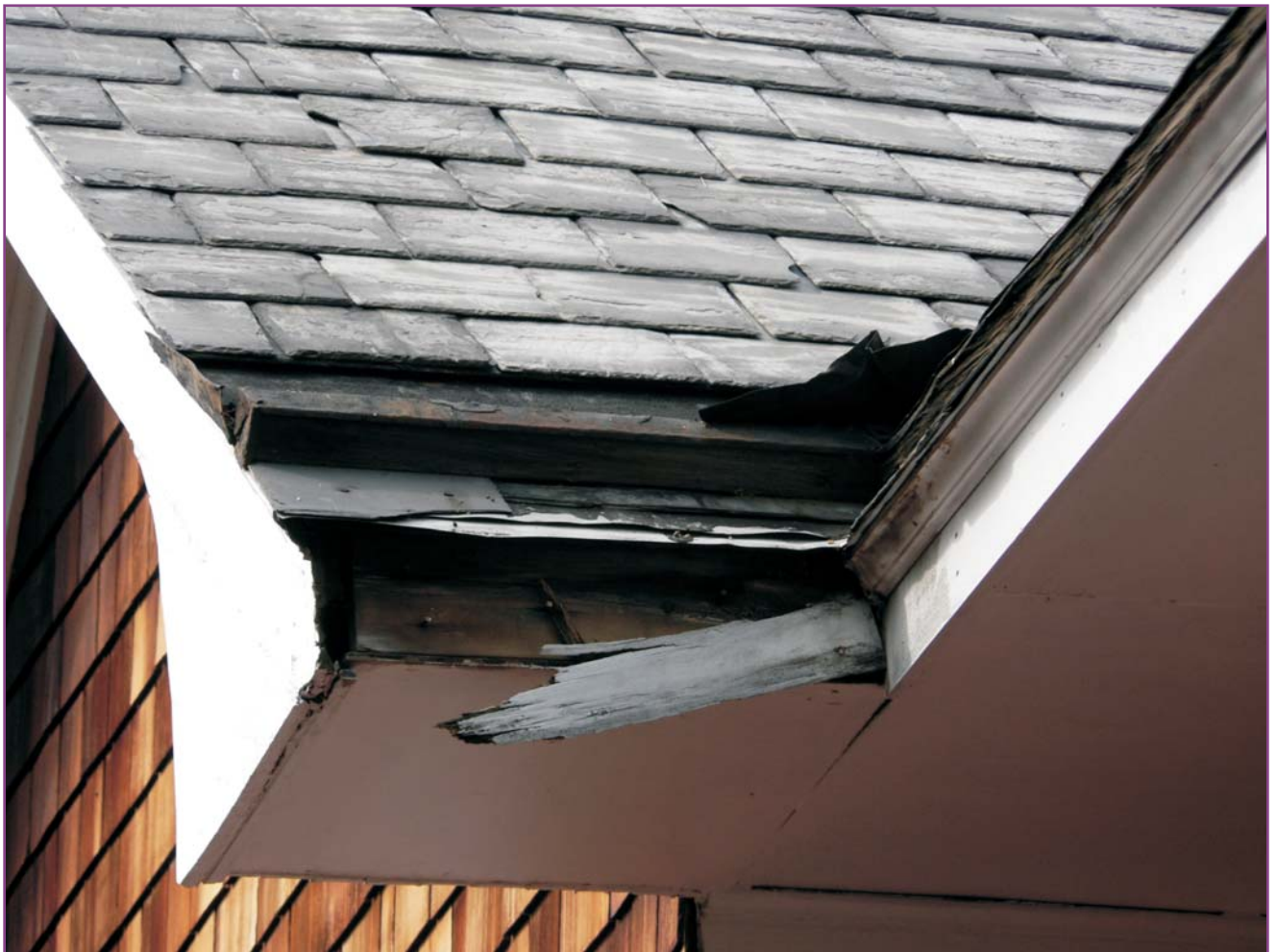
Photograph 26 of 46. Cornice/soffit detail on the southeast elevation (Stanfill Towers side) showing deterioration of the roof slope beneath the pole gutter, loose fascia, and missing cornice woodwork. This is the same area shown in Photograph 18, taken from the attic window, above.
