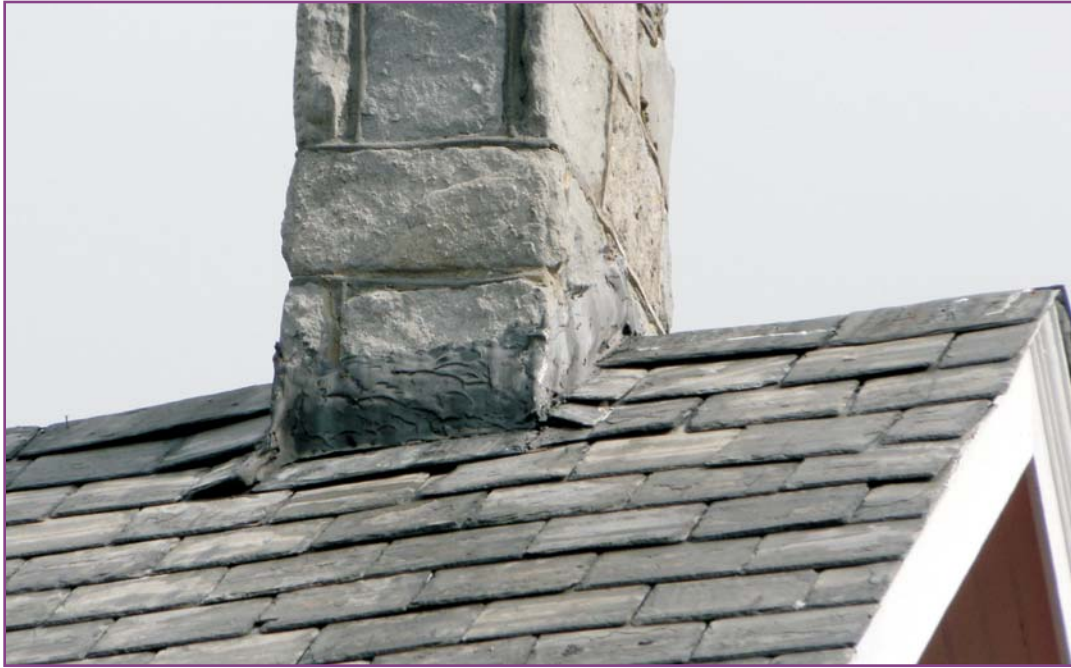
Photograph 19 of 46. Detail of the main chimney at the junction with the front roof slope showing a lack of proper flashing. The original flashing was apparently tin and deteriorated from a lack of re-painting. It appears to have been covered with bitumen (which is incompatible with tin) and allowed further moisture infiltration.
