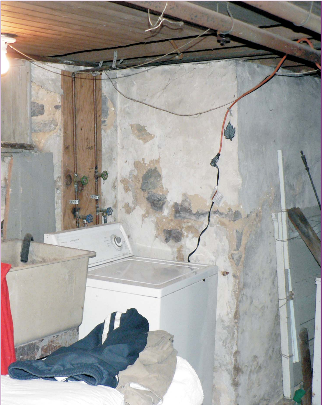
Photograph 37 of 46. Detail of southeastern foundation wall to the rear of the fireplace support showing moisture damage from the chimney leak nearly 30' above, and unsafe use of an extension cord to power the washing machine.
