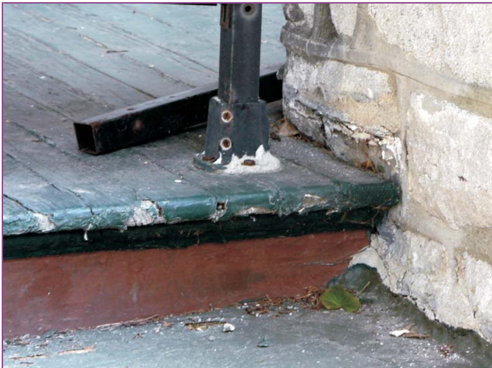
Photograph 5 of 46. Detail of front porch steps at porch pier showing settlement and structural movement. Stabilization of the floor framing will be necessary.
