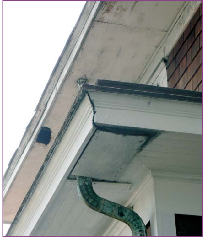
Photograph 29 of 46. Detail of bay and main soffits on northwest elevation (driveway side) showing moisture damage and need for woodwork repairs.
