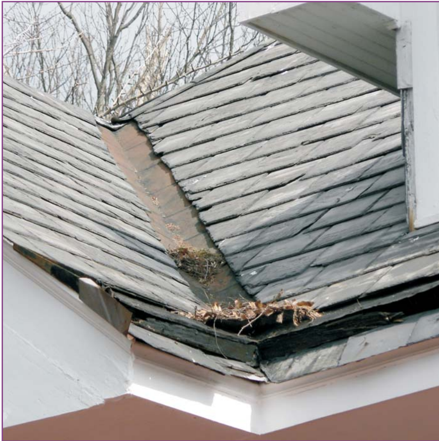
Photograph 16 of 46. Detail of front roof valley showing rusting of the valley flashing, due to lack of maintenance (paint). Note debris and leaves collected at pole gutter.
