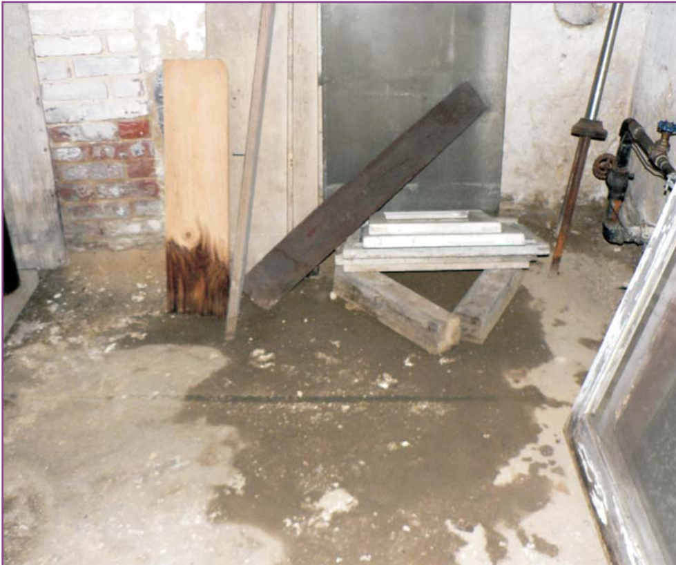
Photograph 45 of 46. Detail of southern corner of basement during rain storm showing water entering despite exterior wrap-around porch in this location.
