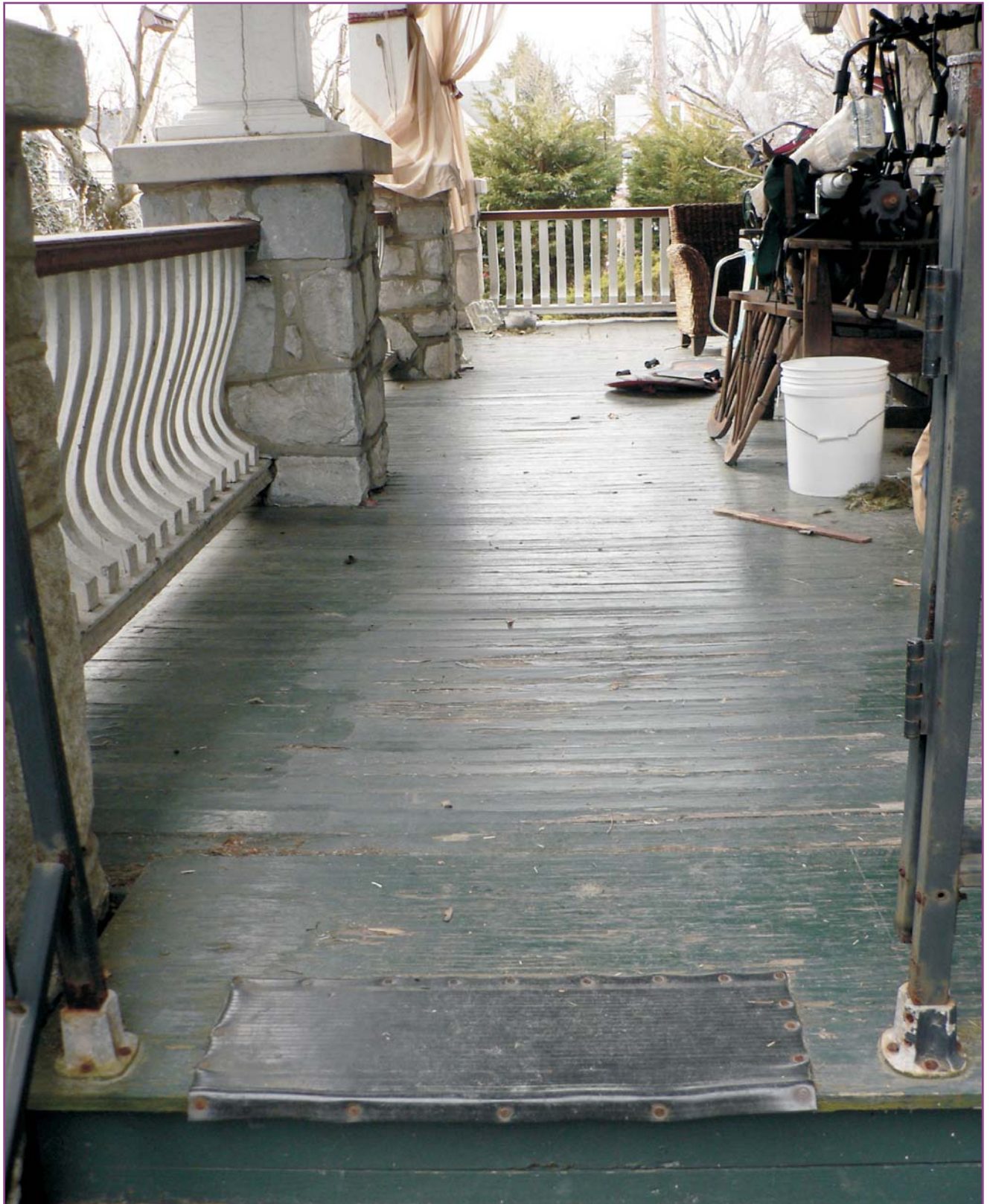
Photograph 8 of 46. View of side return of front porch showing original flooring, balustrade, stone piers, and Doric posts. The metal railing at steps has been added.
