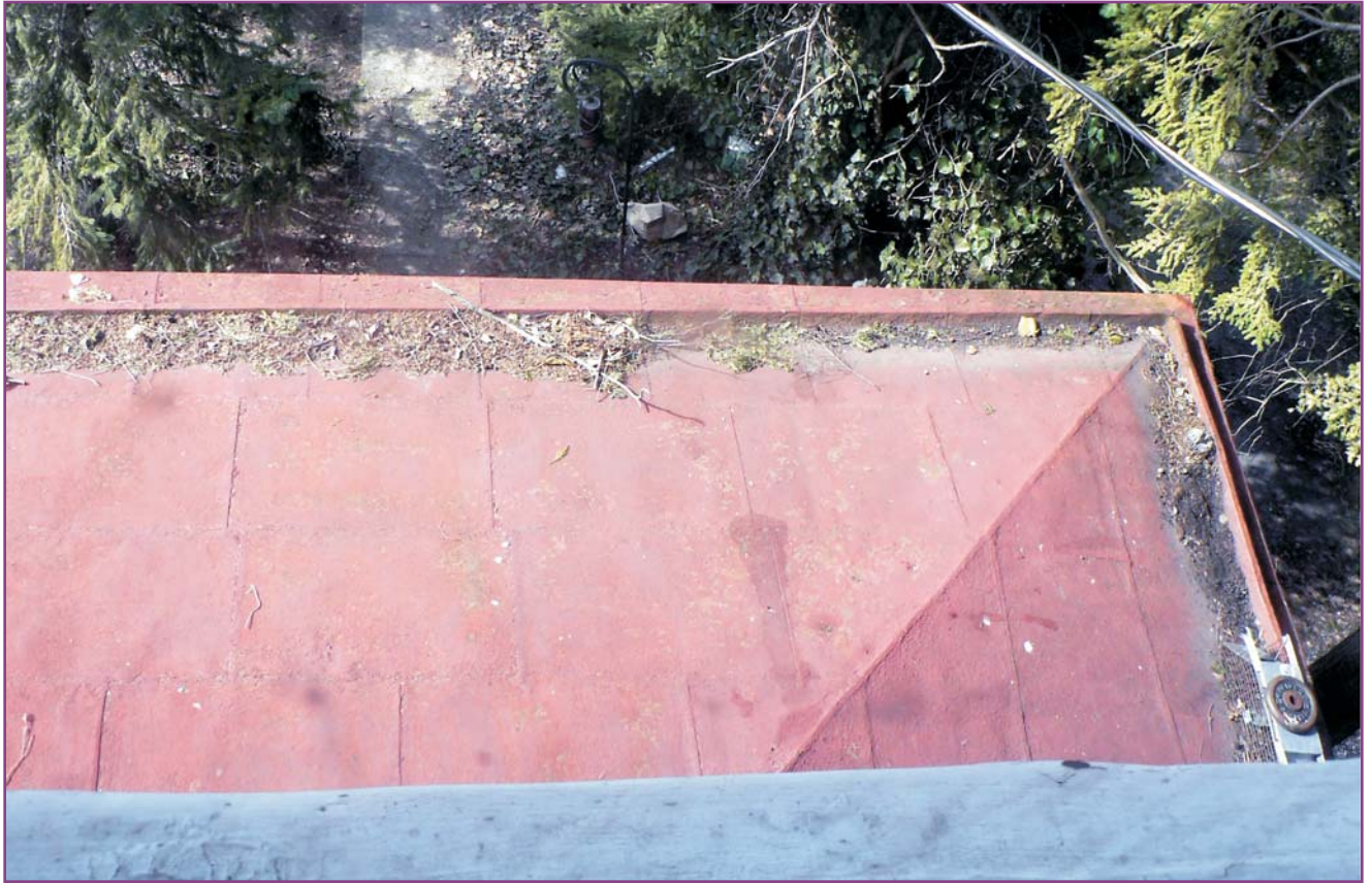
Photograph 11 of 46. View of the porch roof from the attic window. This roof is covered with flat seam metal (terne-plated steel, commonly called tin) that will last forever provided it is kept painted. The “tinner’s red” color is historically appropriate. Note that the pole gutters need cleaning.
