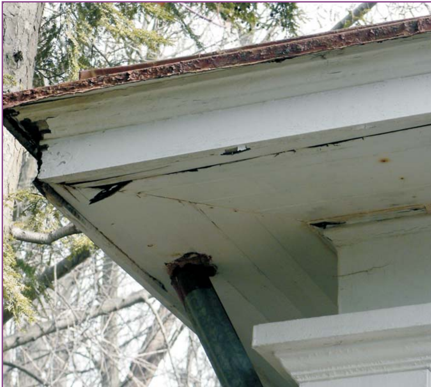
Photograph 12 of 46. Detail of western corner of front porch soffit showing minor woodwork deterioration and failing paint on rusting drip edge.
