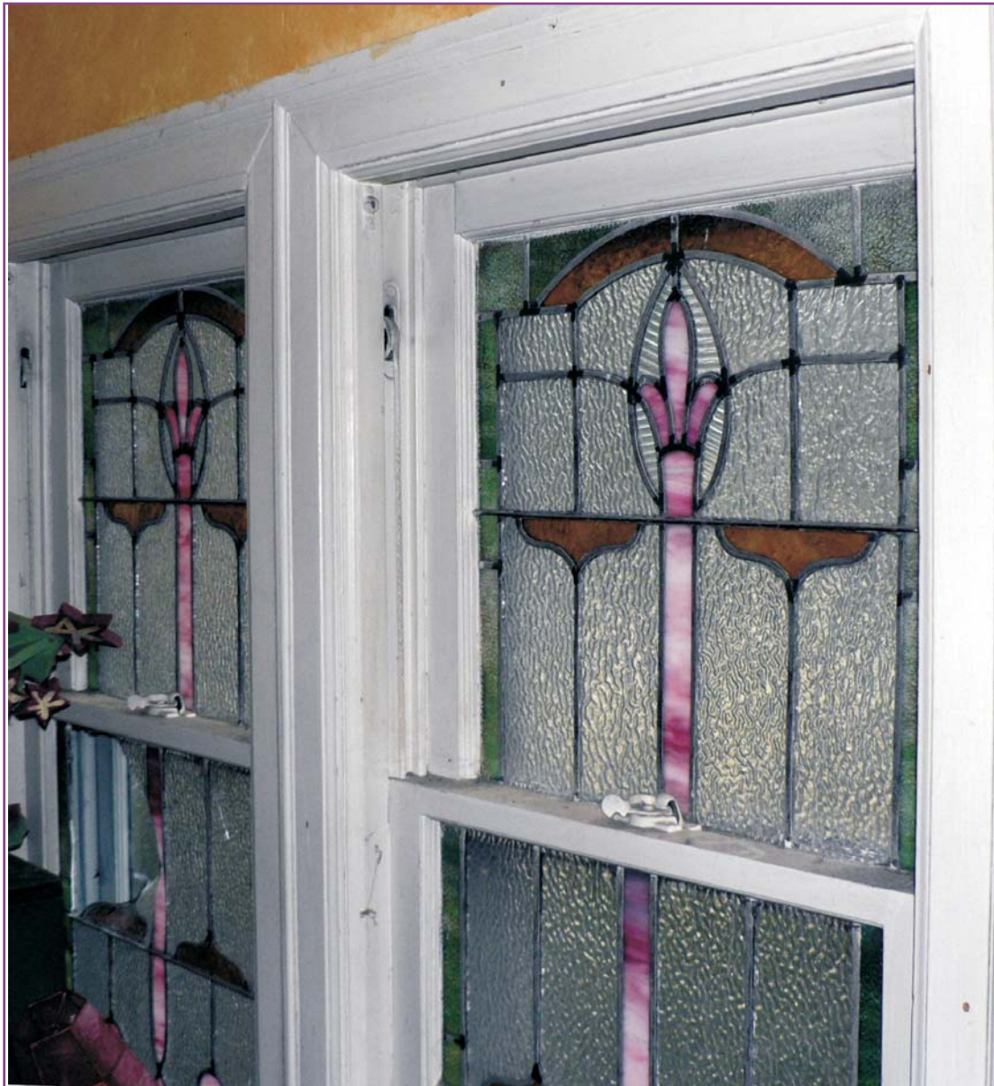
Photograph 46 of 46. Detail of two of the three stained glass windows on the stair landing showing broken section in lower left sash and cracked pane in lower right sash. Note that the intact sash cords on both windows. These sash cords are connected to sash weights hidden inside the window frame that counter balance the bottom sash when the window is opened.
