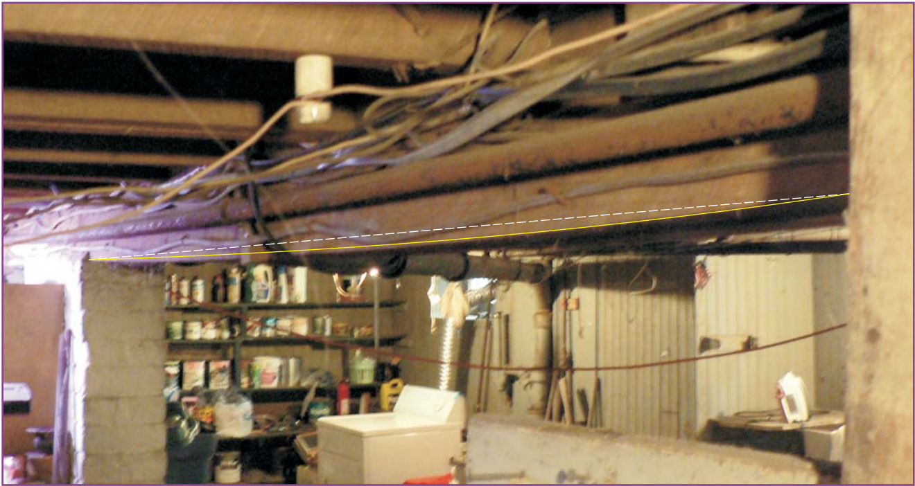
Photograph 40 of 46. View of central structural girder. Note deflection indicated by yellow line. (The white line shows where the bottom of the girder would be if it were level.)
