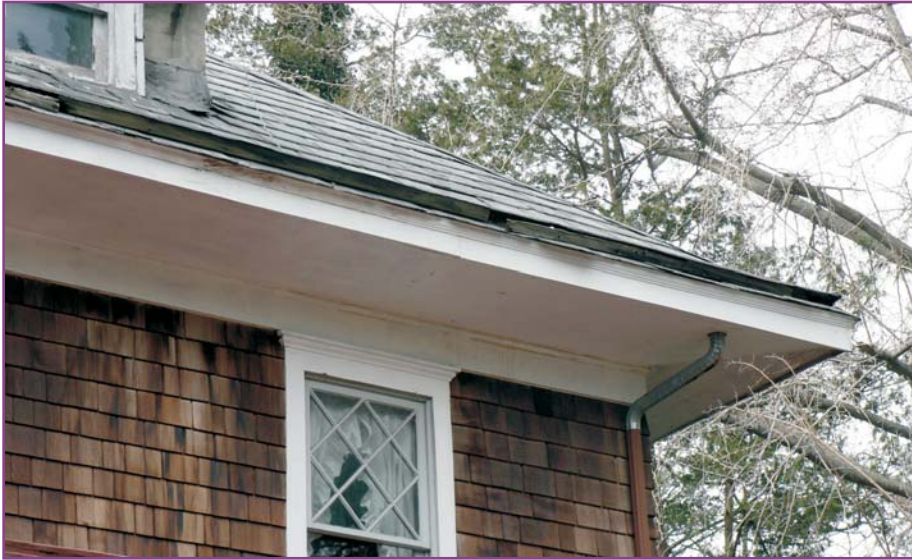
Photograph 24 of 46. Detail of the northwestern end of the rear elevation's roof showing the deteriorated pole gutter.
