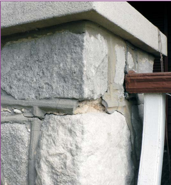
Photograph 7 of 46. Detail of typical stone porch pier in need of spot repointing. Note original cast stone cap and wood balustrade at right.
