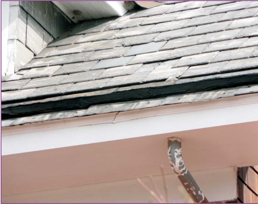
Photograph 17 of 46. Detail of front roof slope showing properly repaired as well as missing slates, rusting pole gutter and downspout, and original slate dormer cheeks which should not be removed when the roof is replaced (because they are sound and will provide evidence of the original roof covering long after it is gone.)
