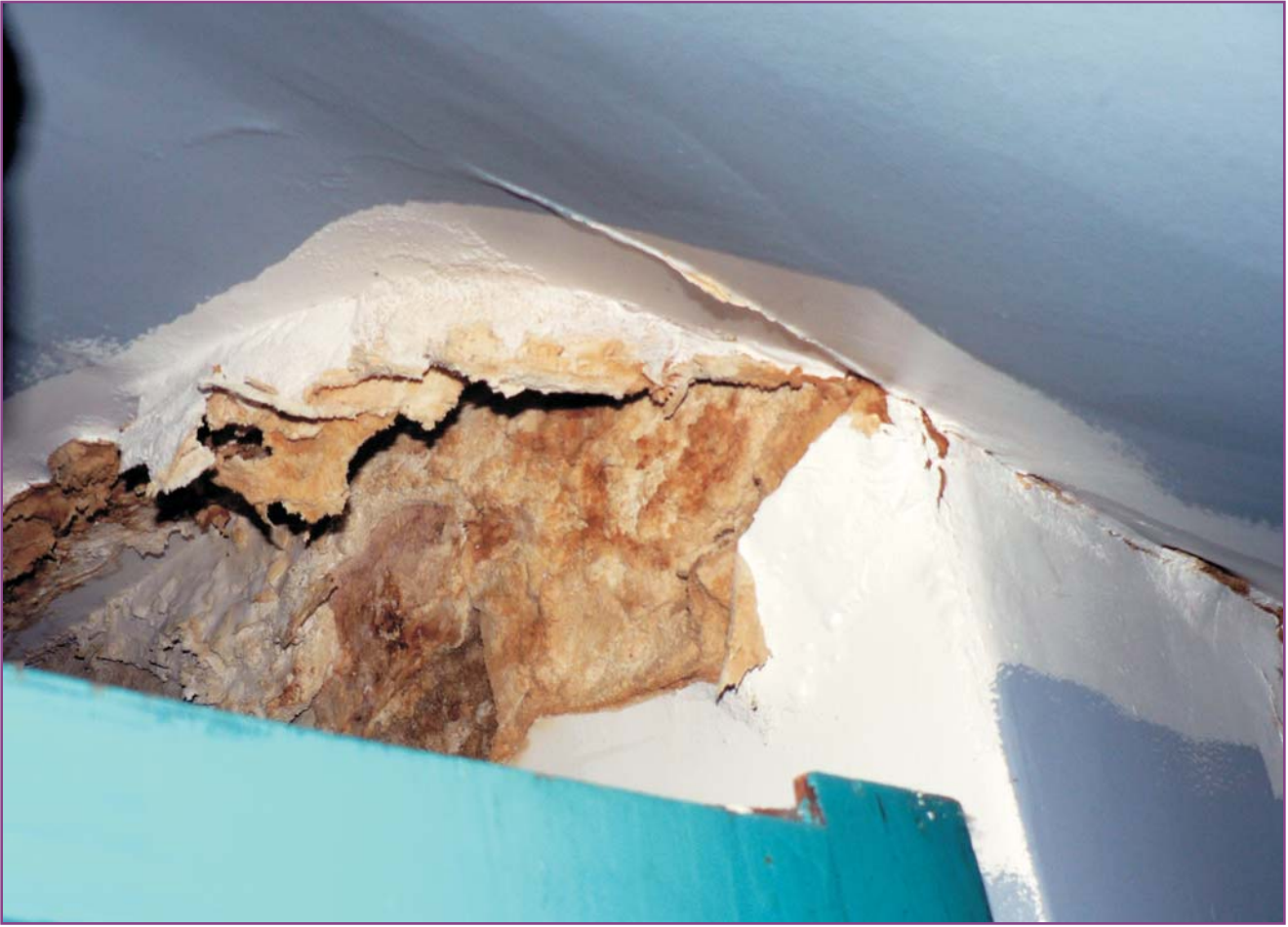
Photograph 21 of 46. Detail of damaged plaster on chimney wall, directly below roof structure and attic ceiling.
