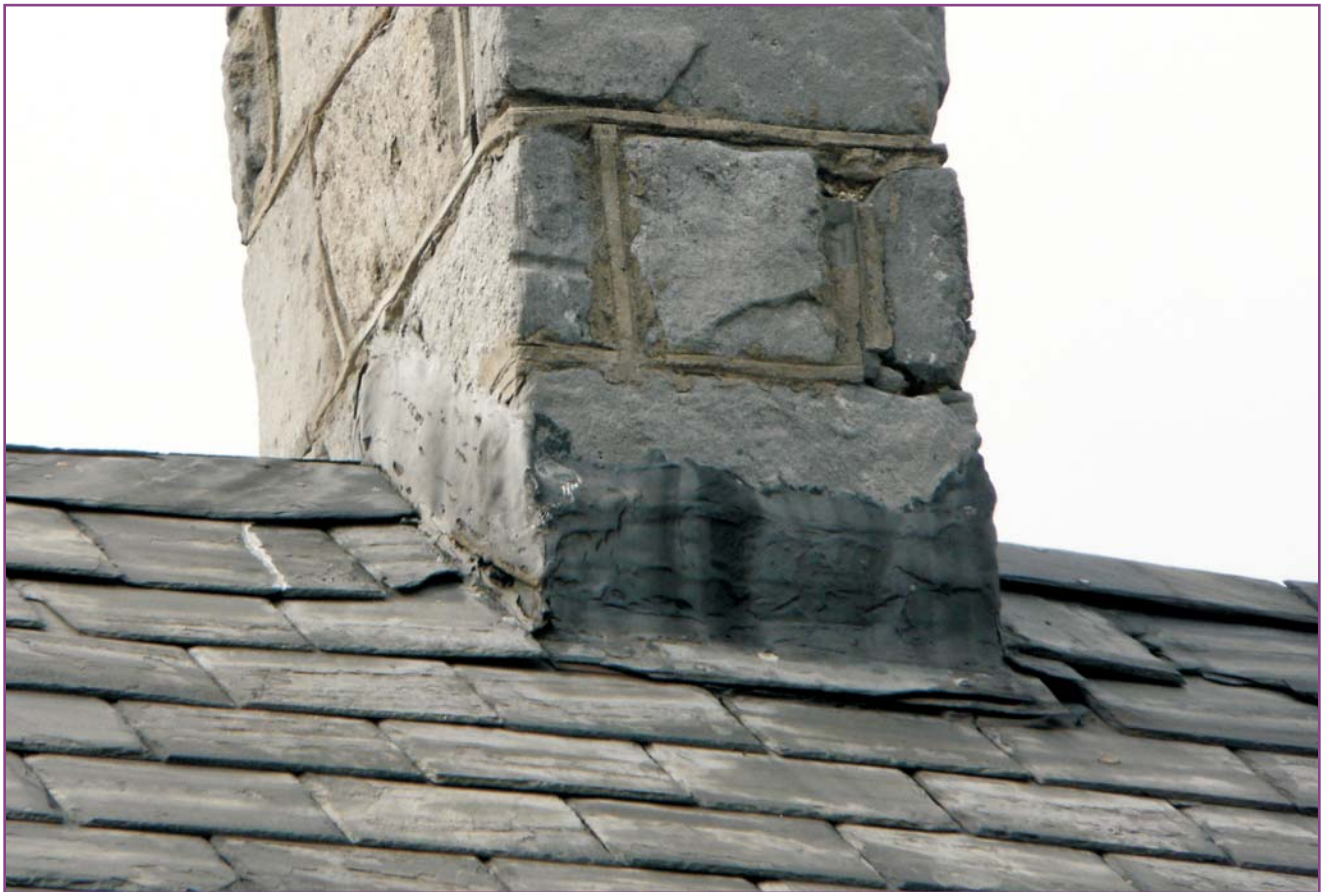
Photograph 20 of 46. Detail of the junction of the main chimney and the rear roof slope showing bitumen-coated flashing and need of spot repointing of the masonry.
