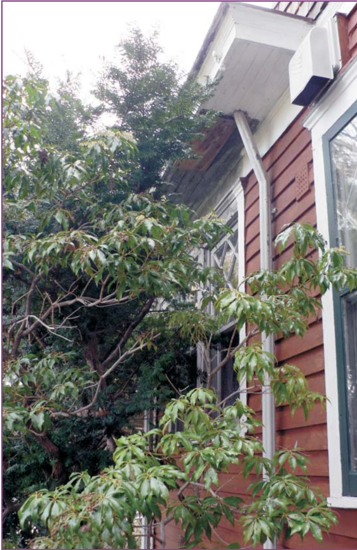
Photograph 30 of 46. Detail of the one story wall of the rear wing on the driveway (northwestern) side showing the encroachment of overgrown vegetation and corresponding deterioration of the woodwork due to the moisture held against the wall by the shrubbery.
