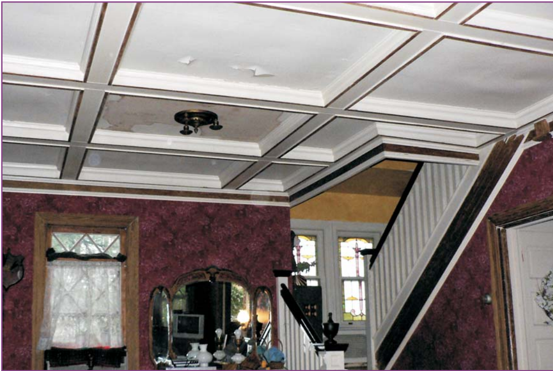
Photograph 34 of 46. View of first floor living room showing coffered ceiling. There is significant paint peeling on this ceiling; however it appears to be an aesthetic issue due to the paint's age, not a sign of water infiltration.
