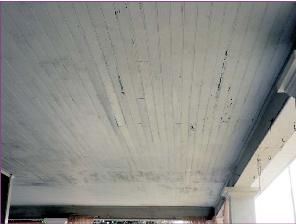
Photograph 10 of 46. Detail of front porch's beaded board ceiling showing buckled board and peeling paint at small leak.
