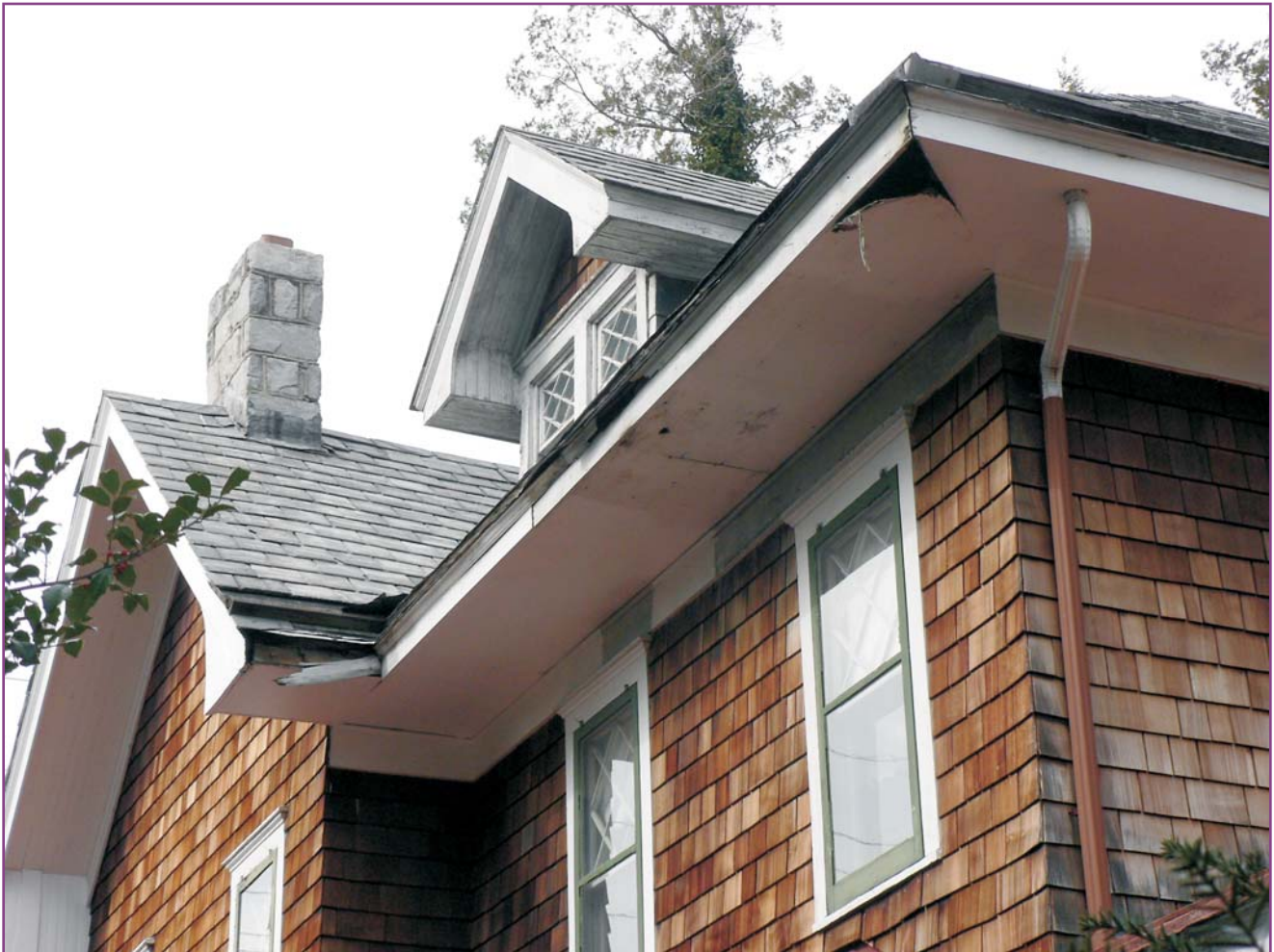
Photograph 25 of 46. View of the soffits and side cross-gable of the southeast elevation, viewed from the rear yard. Note hole in soffit.
