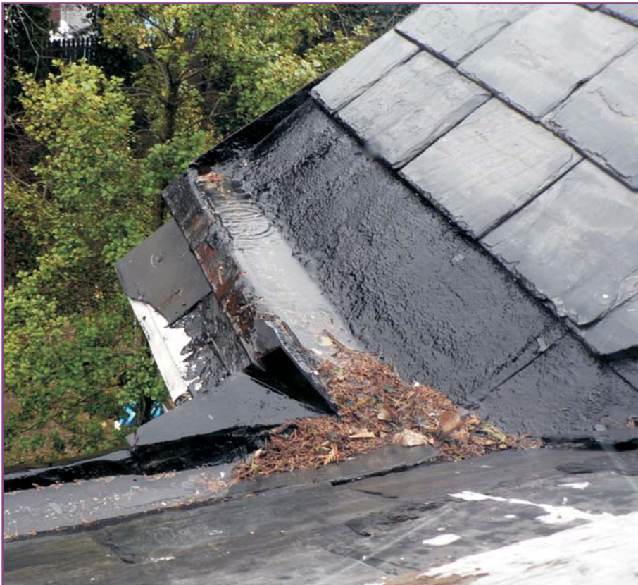
Photograph 18 of 46. Detail of slate condition on southeastern side roof as seen from attic window. Note water running over the top of the clogged pole gutter causing deterioration to the woodwork of the cornice below.
