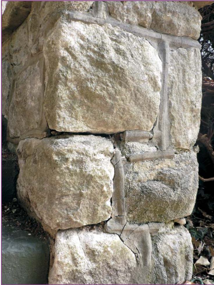
Photograph 4 of 46. Detail of southern cheek wall at front steps showing masonry movement in response to deteriorated mortar joints. Repair and spot repointing is required.
