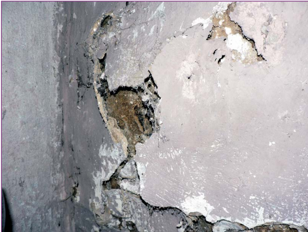
Photograph 43 of 46. Detail of exfoliating plaster caused by water entering the basement foundation walls.
