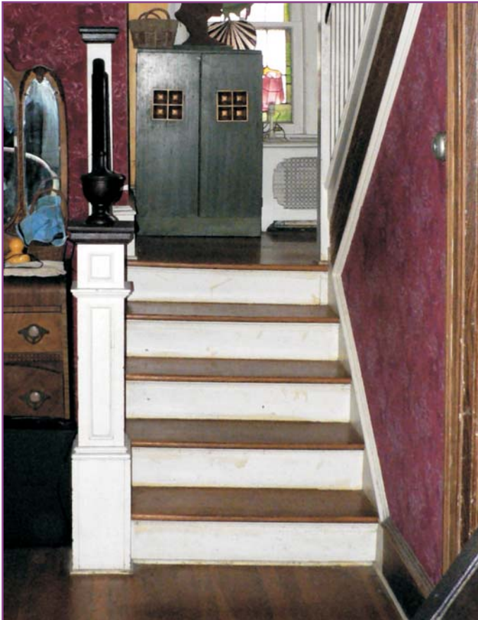
Photograph 35 of 46. Detail of living room stairs showing settlement of steps towards the center wall. There is a corresponding depression of the floor in the adjacent music room. Both are the result of the failed beam shown in basement photographs 40 and 41.
