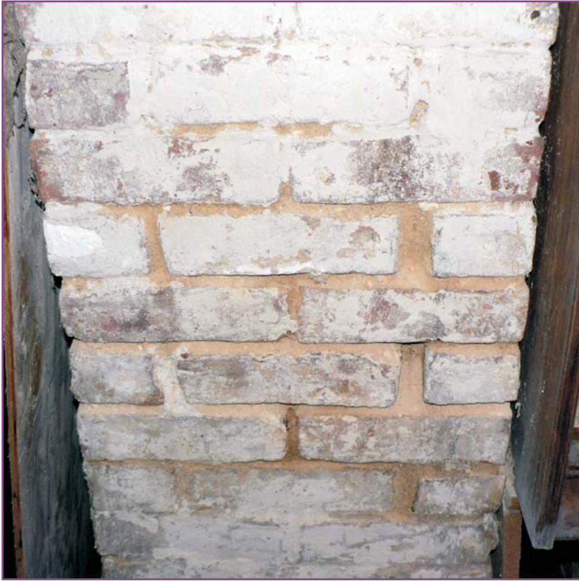
Photograph 44 of 46. Detail of typical brick pier in basement in need of spot repointing.
