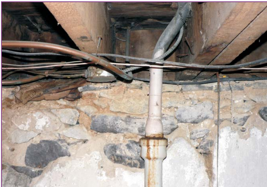
Photograph 39 of 46. Detail of typical area of moisture damage at the top of the foundation walls. Both the plaster and the mortar joints have deteriorated, and the wood framing is stained.
