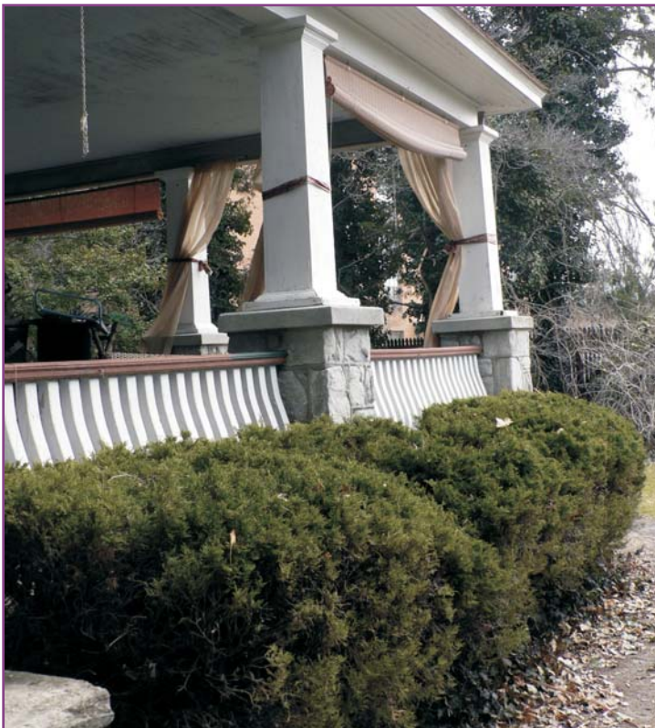
Photograph 3 of 46. View along front porch showing proximity of overgrown bushes that hold moisture against the porch's stone foundations. These bushes need to be pruned.
