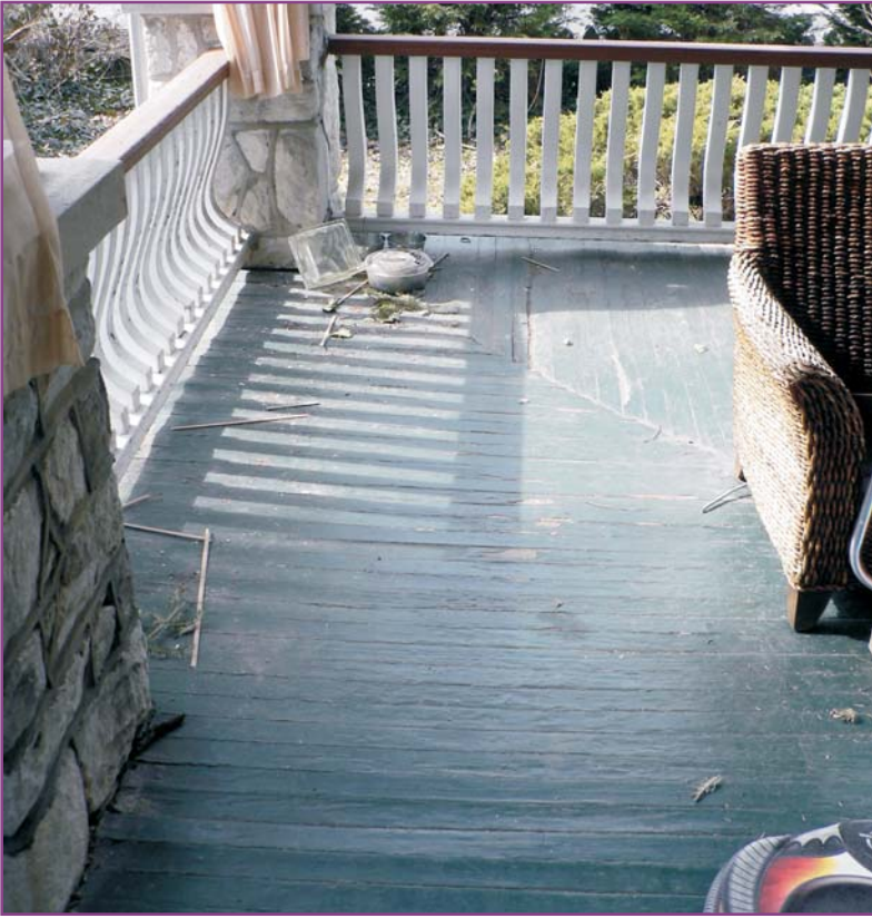
Photograph 9 of 46. Detail of southern corner of front porch floor showing depression at failed floor framing. This framing will need to be stabilized.
