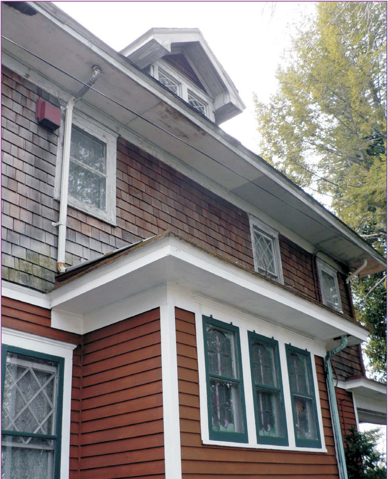
Photograph 27 of 46. View of northwest elevation (driveway-side wall) at box bay of stair landing showing failure of the downspout where it meets the bay's roof and broken stained glass in far first-floor window. (Also shown from the interior in Photograph 46.)
