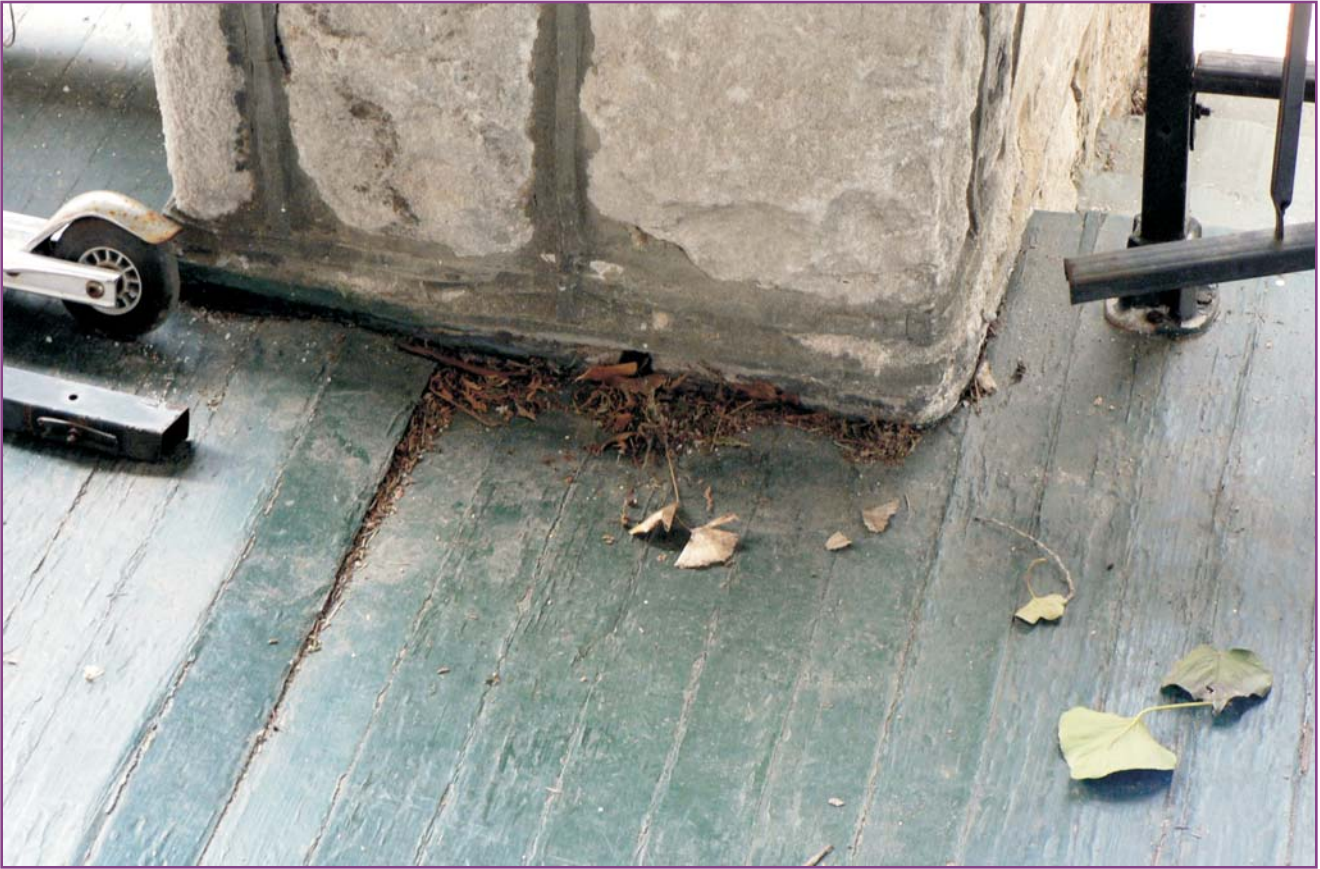
Photograph 6 of 46. Detail of same porch pier (from porch side) showing settlement.
