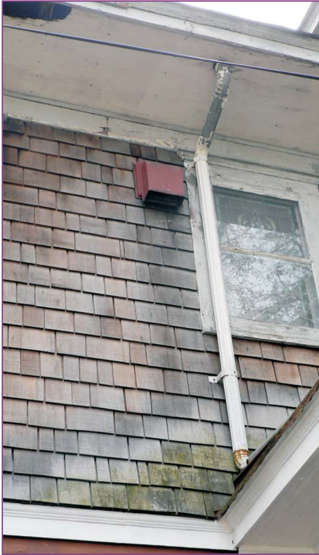
Photograph 28 of 46. Detail of the downspout failure showing organic growth on the wall shingles due to excessive dampness.
