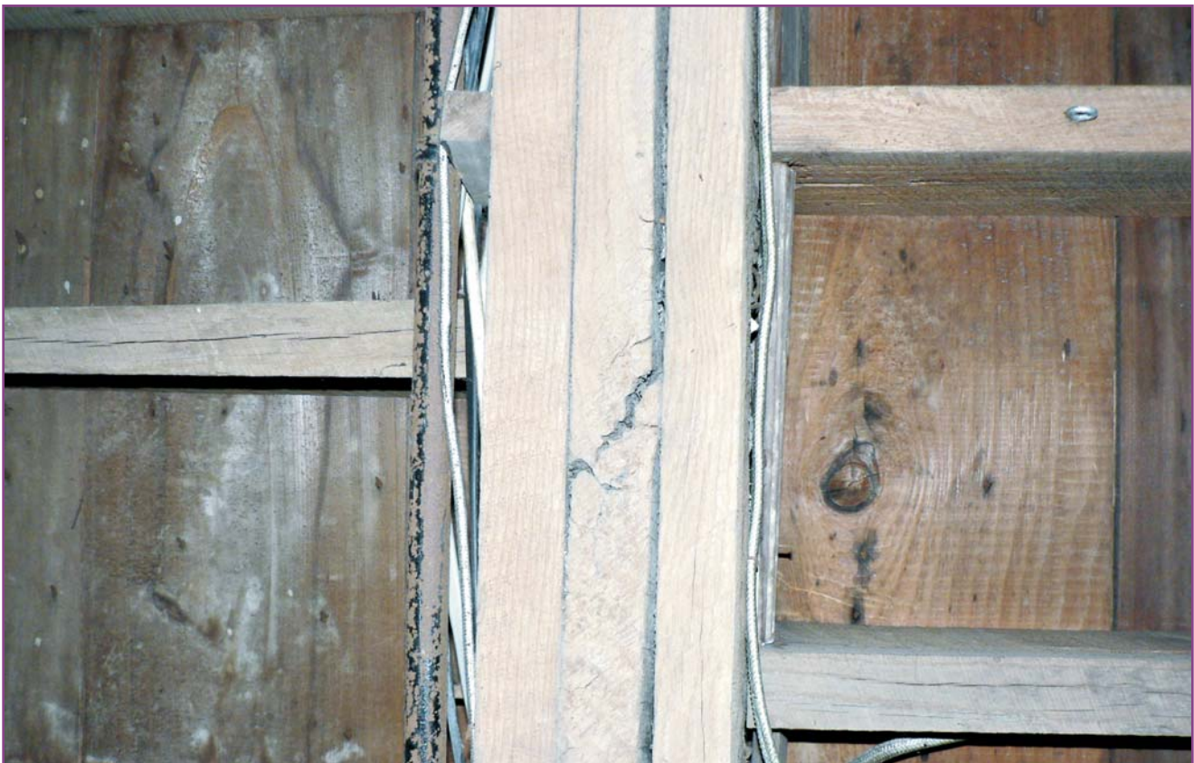
Photograph 41 of 46. Detail of partially failed central built-up girder.
